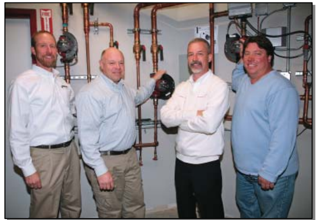
(Left to right) Randy Schaefer, president of WMS sales; Henry Kroll, Orange County Choppers; Dan Fletcher, Grundfos sales agent; and Larry Krug, Orange County Sheet Metal, were all involved with the installation of several Grundfos MAGNA circulators inside the mechanical room at OCC.
